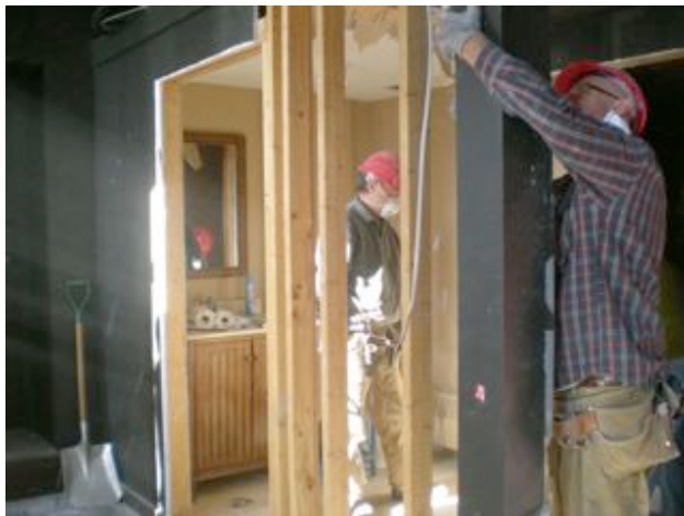
Dave Clark and Dave McTavish remove the wall to create a new washroom hall.
